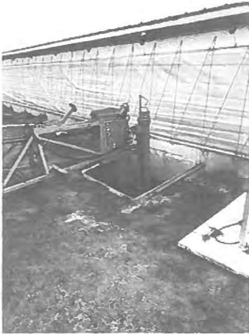
5. A pump-out with ventilation fan removed for agitation during manure application.
