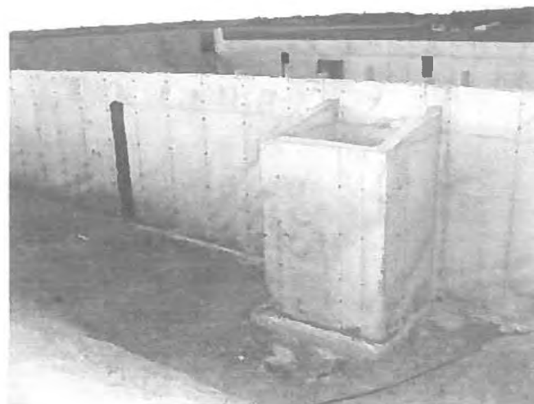
4. Each fall, waste is pumped out of five 5'x6' pump-outs.
