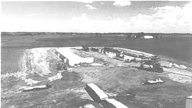
1. This photo shows the first of two identical pollution control devices, including slats on truck.
